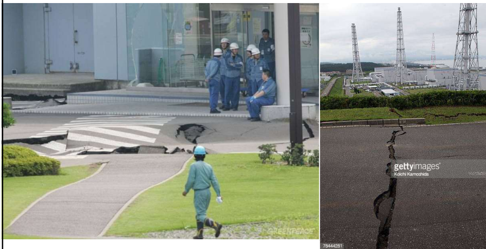
Kashiwazaki Kariwa NPP: fractures on the surface of the site and damaged access road.
